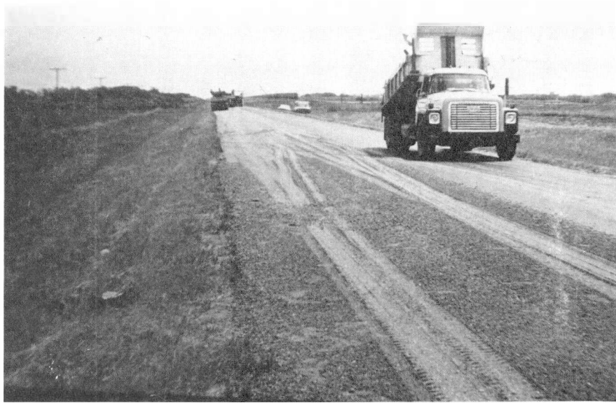
Maintenance Truck Provided Gravel for Missed Patches
