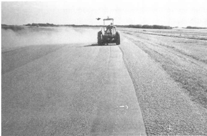
Brooming of C.S. 9-2 Showing Excess Aggregate
