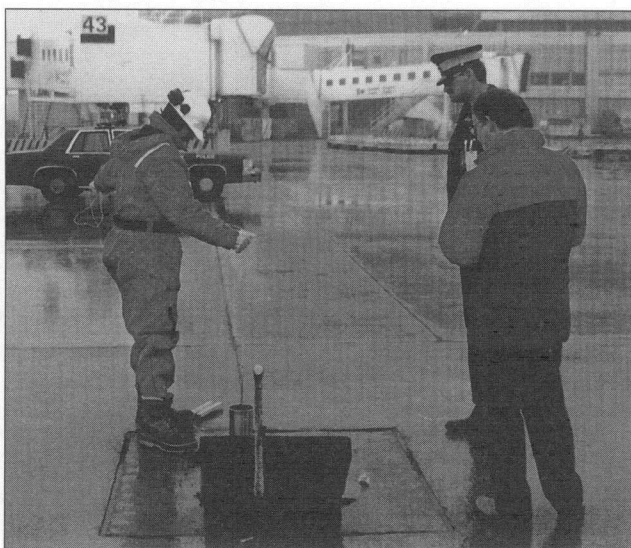
Inspecting a glycol leak at Toronto's Pearson Airport.
