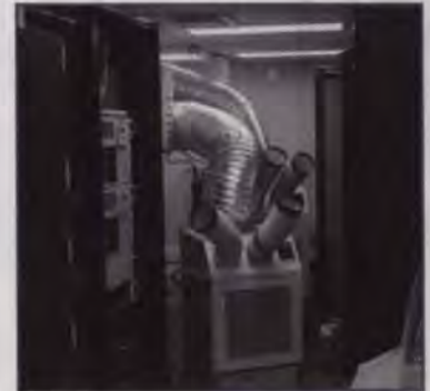
Emergency portable air conditioners in server room
