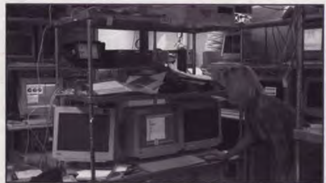
Network Operations Centre at C.D. Howe
