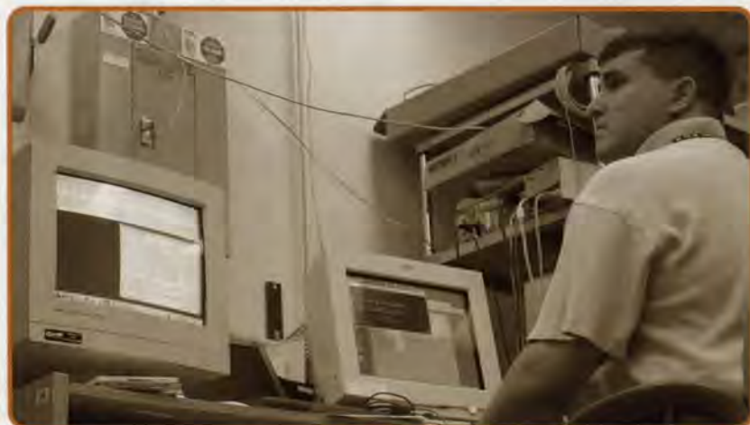
C.D. Howe Server Room.
