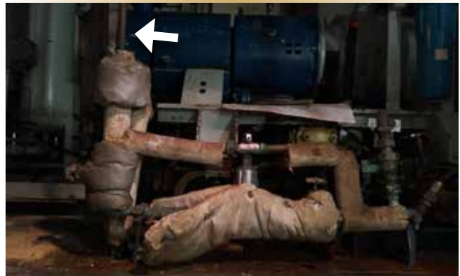
Figure 3. Flex line to LPA compressor cooling.
