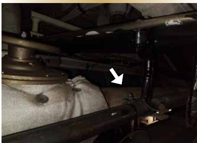
Figure 6. ASWC supply in the forward engine room.
