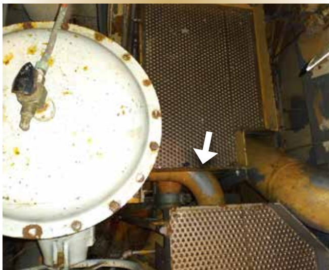
Figure 5. The auxiliary seawater circulation (ASWC) system supply in the after engine room.
