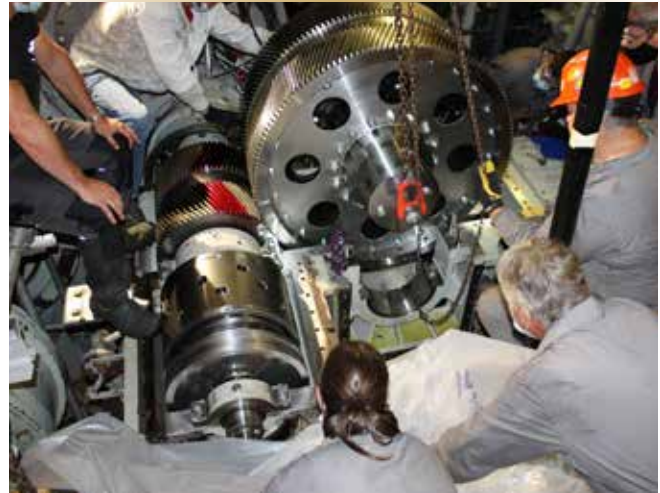
Figure 4. Formation gearing inspectors Patti Fraser and Stephane Chouinard observe the installation of the new gear.
