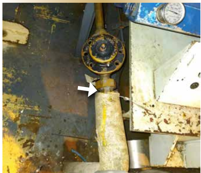
Figure 4. Flex line to the chilled-water return main.
