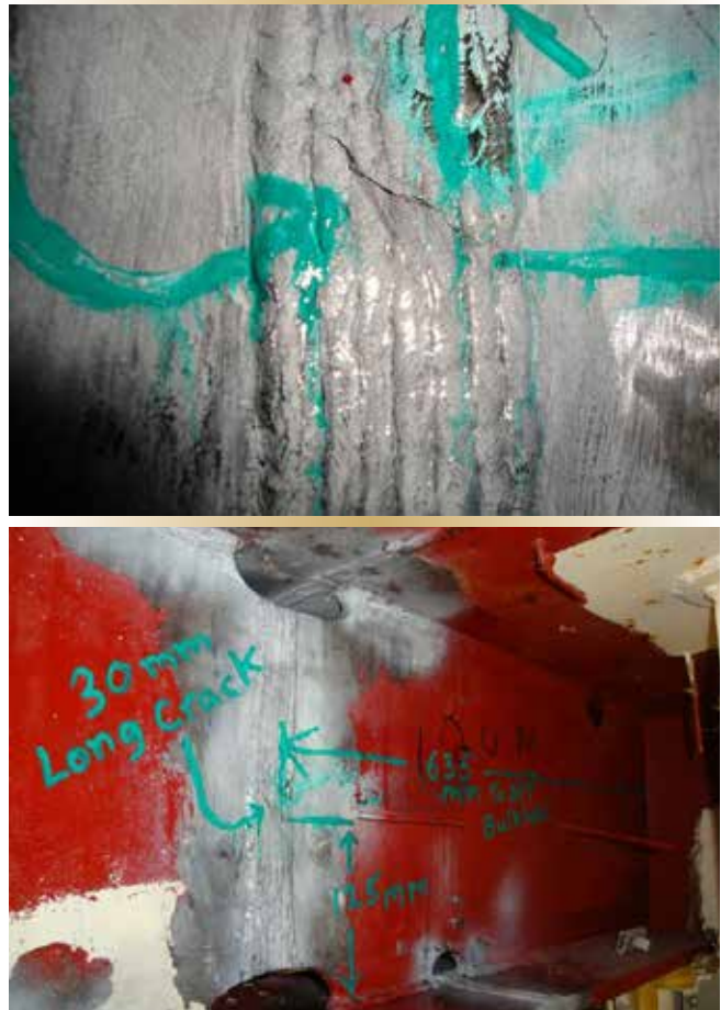
Figure 3. A 30-mm crack found on the web of a girder aboard HMCS Ville de Québec (FFH-332). (Huang, 2021)
