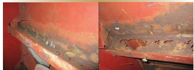
Figure 2. Holed and wasted sections of longitudinal.
