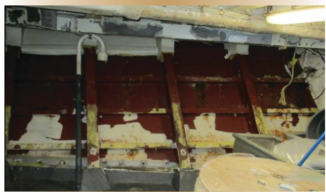
Figure 1. Area of corroded steelwork on the port side of the foc'sle mezzanine deck.
