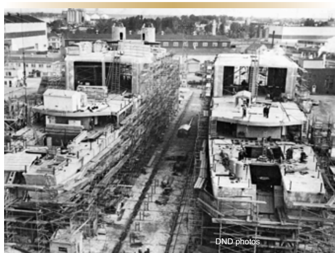
The DDH-280 Tribal-class destroyers Iroquois (left) and Huron under construction at Marine Industries Ltd., Sorel-Tracy, Québec circa 1970.
