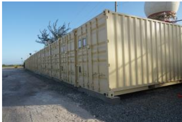
12 - The new Sea Containers were placed on concrete blocks after completion of the TEU Pad.
