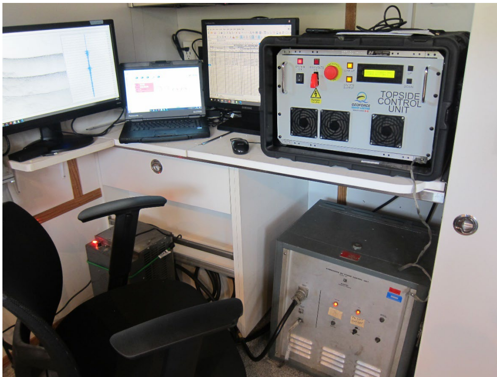
Figure 6 - DTS Topside equipment in operation
