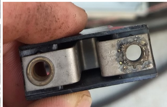
Figure 9 - Thermal Cutout result of arcing
