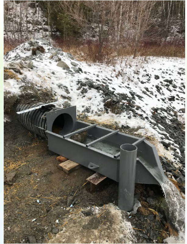
H-Flume at Shaft #98
