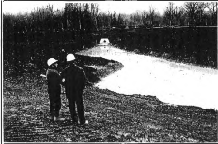
Figure 16 Stormwater Pond in Ajax, Ontario - pond site located in valley adjacent to ESA - during construction
