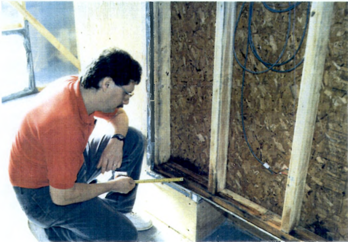
Photo 9 Wood rot at bottom of test panel F (typical of all panels).
