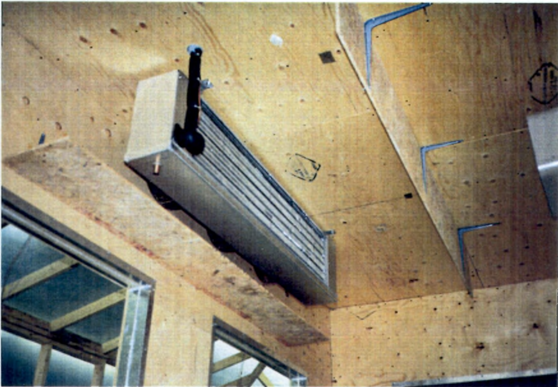
Photo 3 View of refrigeration coil with fan baffles in chamber
