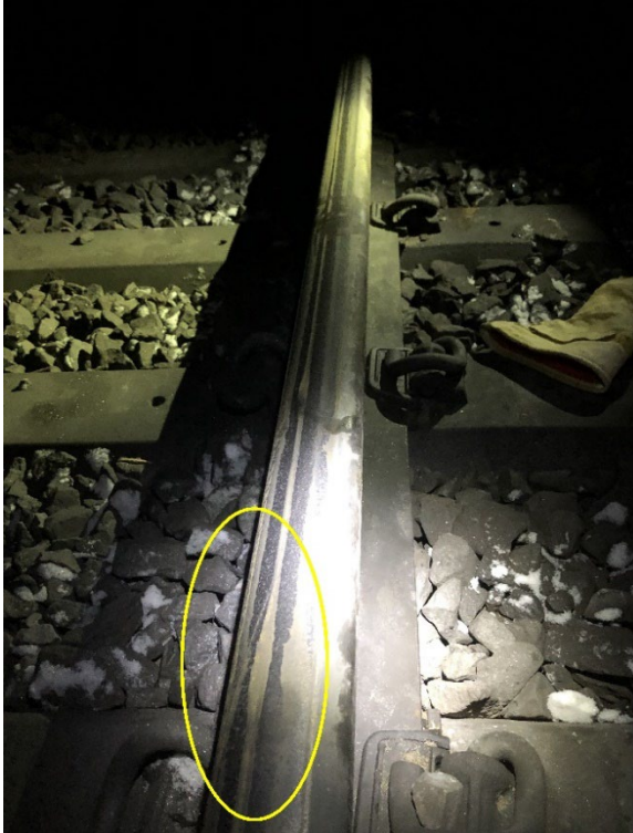
Figure 5. Wheel flange mark (circled) indicating that a wheel had climbed up and over the outside rail (Source: Canadian Pacific, with TSB annotations)
