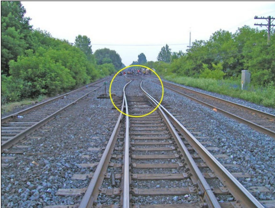
Figure 7. Track buckle (Source: TSB Railway Investigation Report R05H0013)
