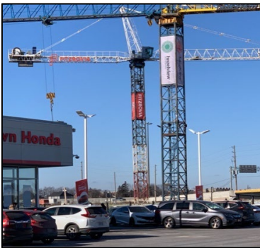
Figure 5: Image of Purpose-Built Rental Construction Site Owned by Hazelview Investments, AIMco, & Fitzrovia Capital (Dufferin and Highway 401)
