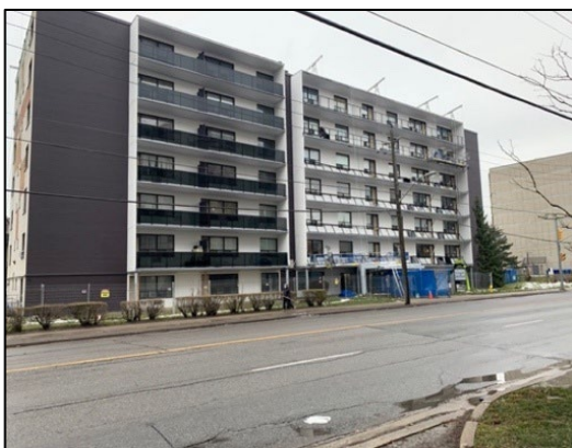
Figure 3: Photo of Exterior (balcony panel replacement) Value-Added Strategy by Starlight Investments in Toronto
