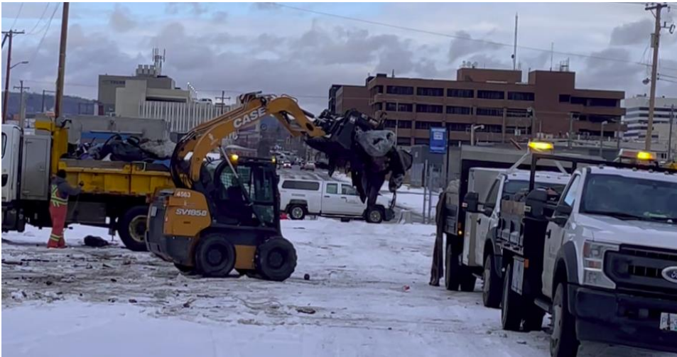
Figure 4: A front-loading bobcat operated by City of Prince George staff loads debris from demolished shelters into city trucks. Still image (at 46 seconds) from video Exhibit B, The 7th Affidavit of Michelle McGregor, File number iMG_9670_MOV Dec 7, 2021. File No. 2160169, Prince George Registry.
