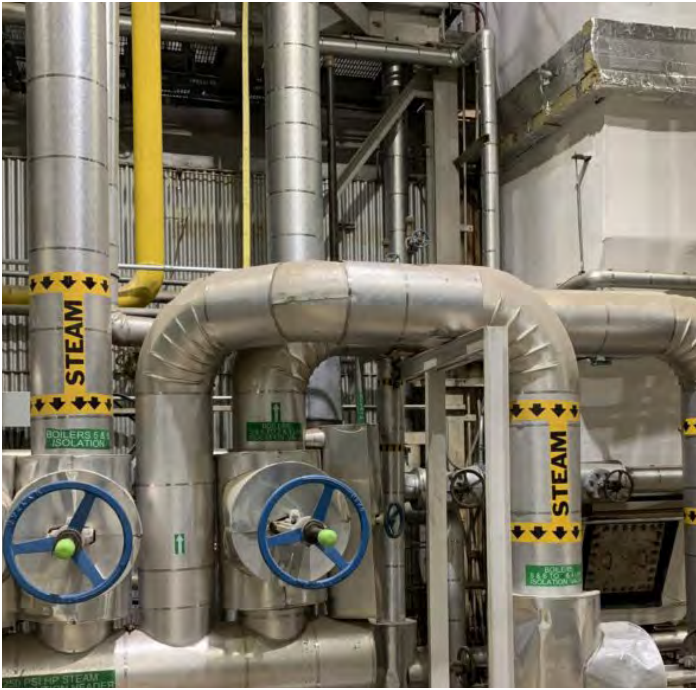
» Markham District Energy
