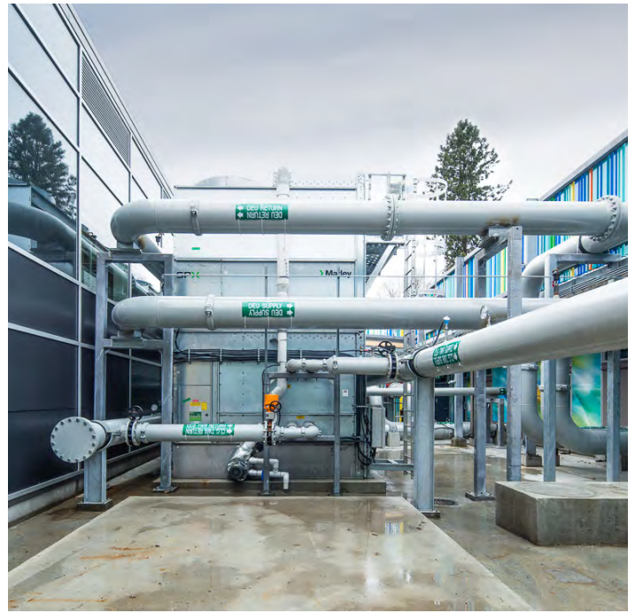
» Lulu Island Energy Company et Corix Infrastructure Inc.
