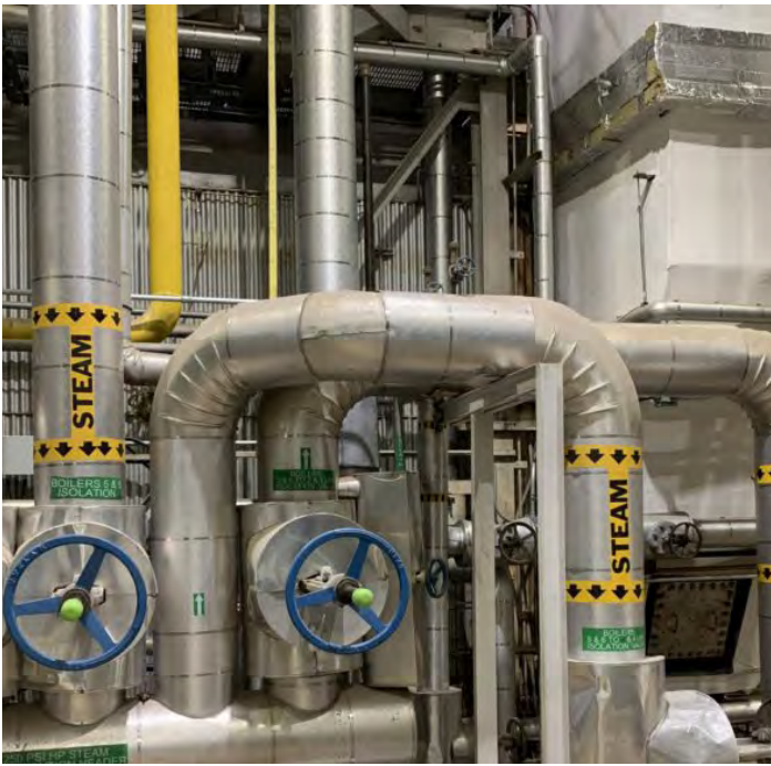
» Markham District Energy
