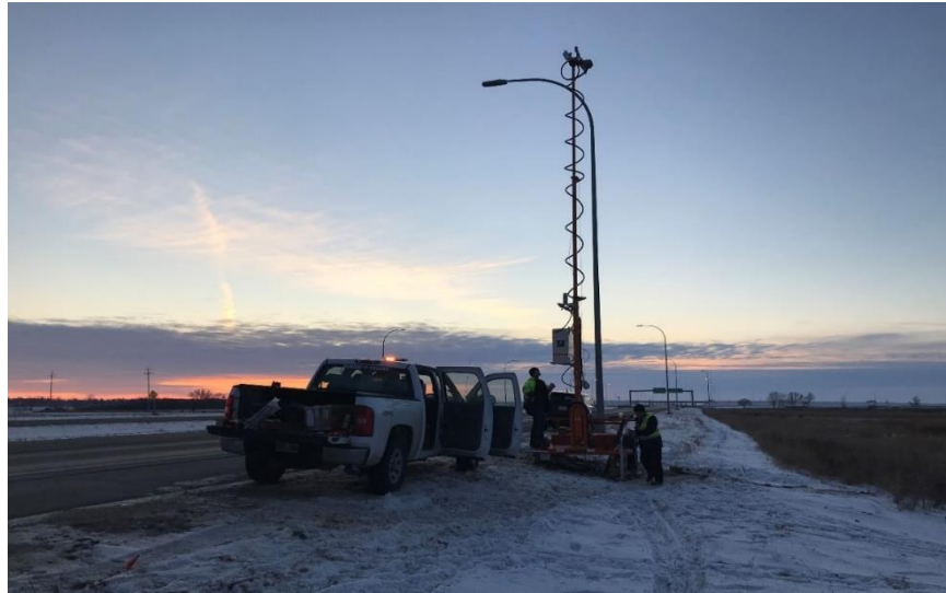
Initial deployment of a portable road-weather and traffic information system in Manitoba
