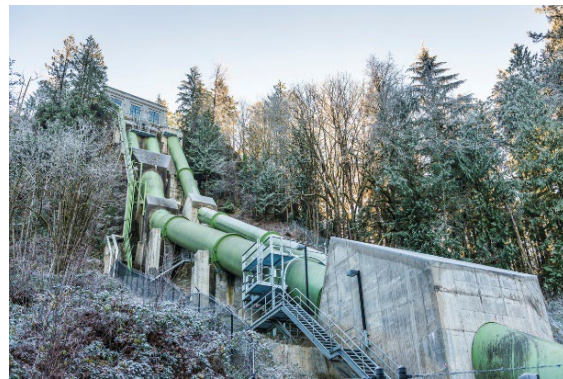
(b) Close-up of penstocks at Snoqualmie power station (iStock.com/Joecho-16)
