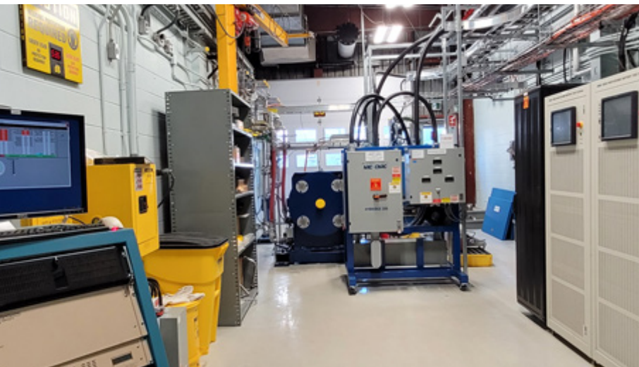
Equipment overview of the Hybrid-Electric Research Outfit facility.
