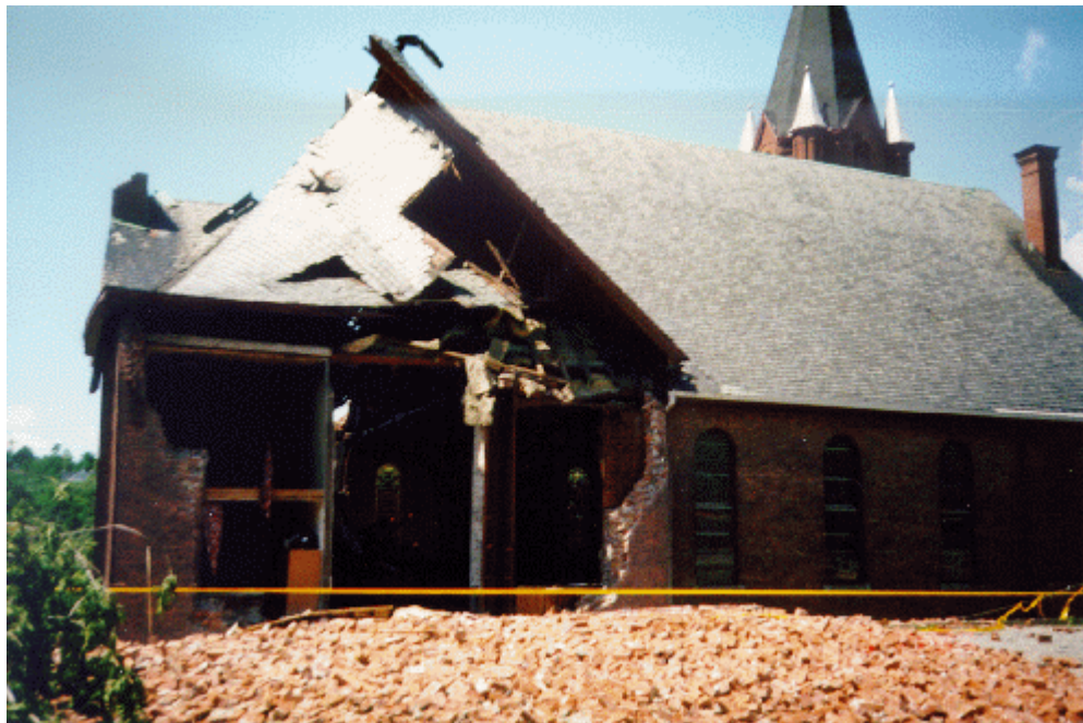
Photo 2 – East side of St. Andrew church, with remains of brick wall downwind
