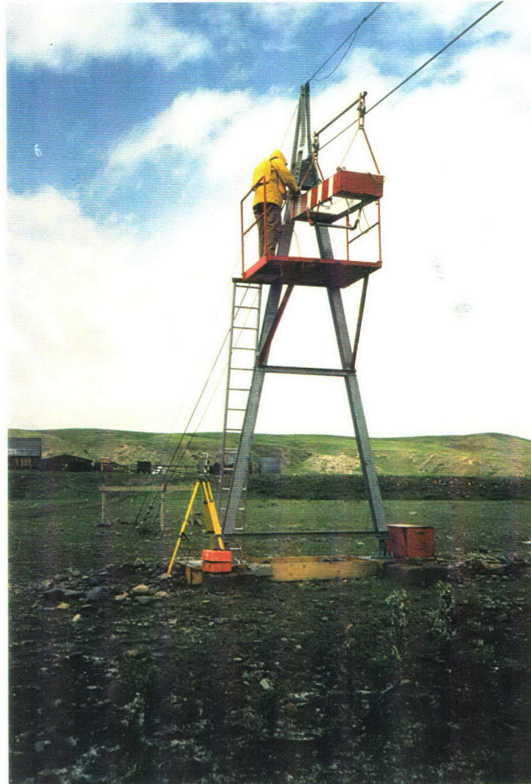
St. Mary River at International Boundary New 20 foot galvanized tower, 7/8" main cable, and right bank deadman installed (3/Jun/1998)
