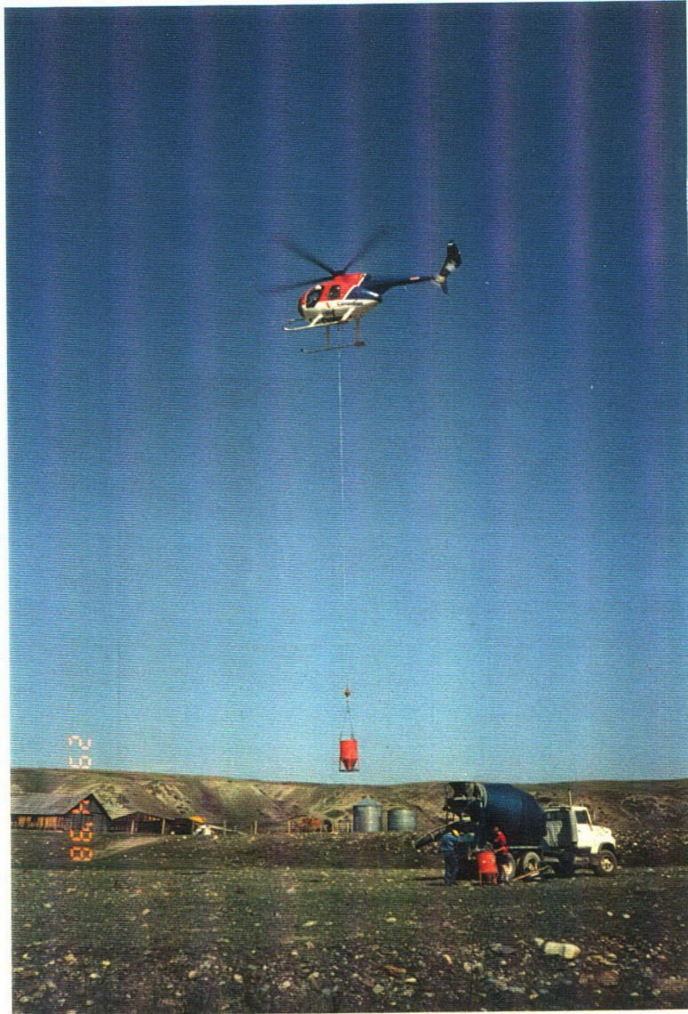
St.Mary River at International Boundary Another load of cement lifting off for The right bank deadman. 29, April, 1998
