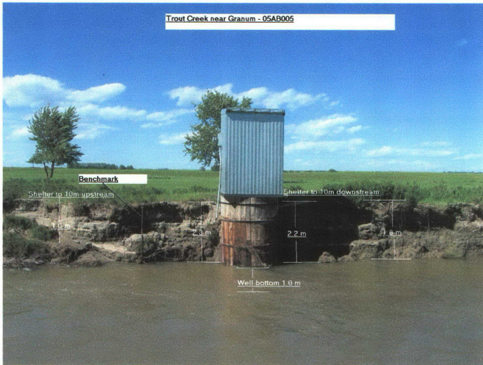
Figure 1: Trout Creek Granum – 05AB005 Flood Damage
