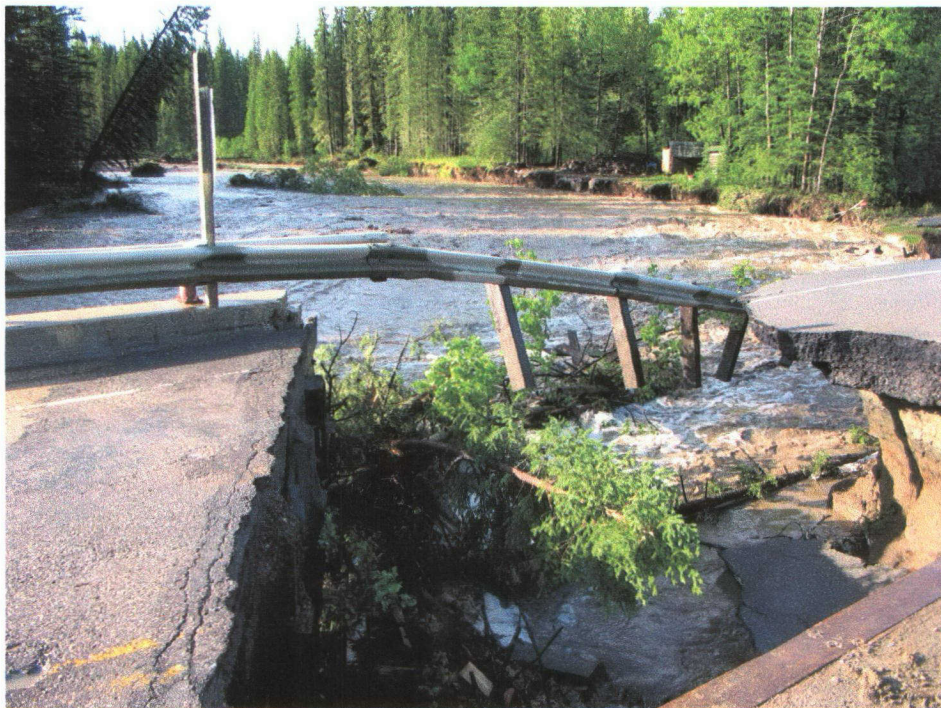
Figure 2: Prairie at Lick Creek flood damage, June 2005
