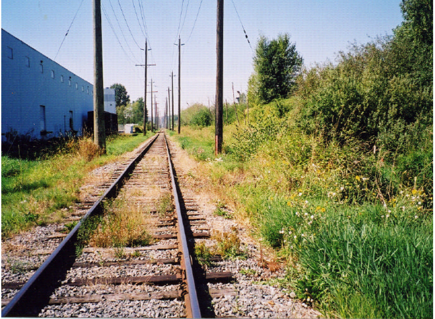
Figure 3. CP Rail Burnaby M11.95 ( 49^{\circ} 12.157' – 123^{\circ} 00.758' ); 10 m PFZ , at a creek crossing below railway; red marker shows adjacent ROW ditch
