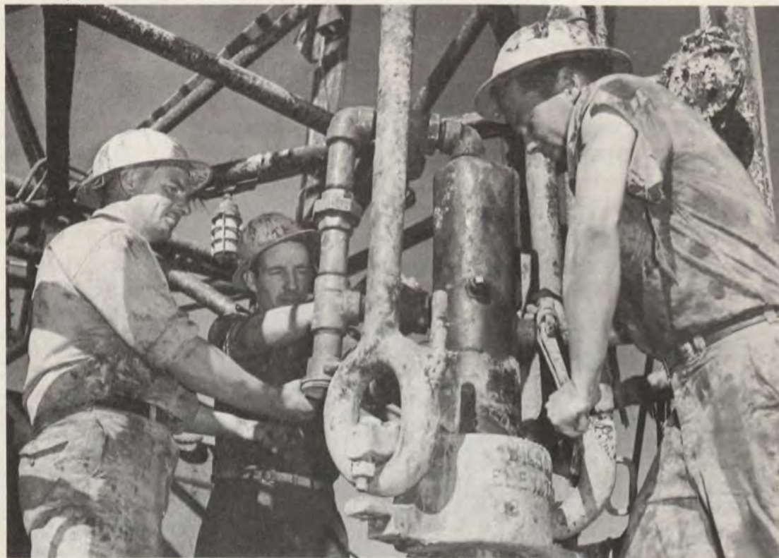
At Imperial Oil Well No. 34 at Redwater, Alberta, the driller, who handles the lead tongs, and the cathead operator release pressure off the casing on the cement head. Cement is poured down the 7-inch casing and, by pressure, up around the pipe.
