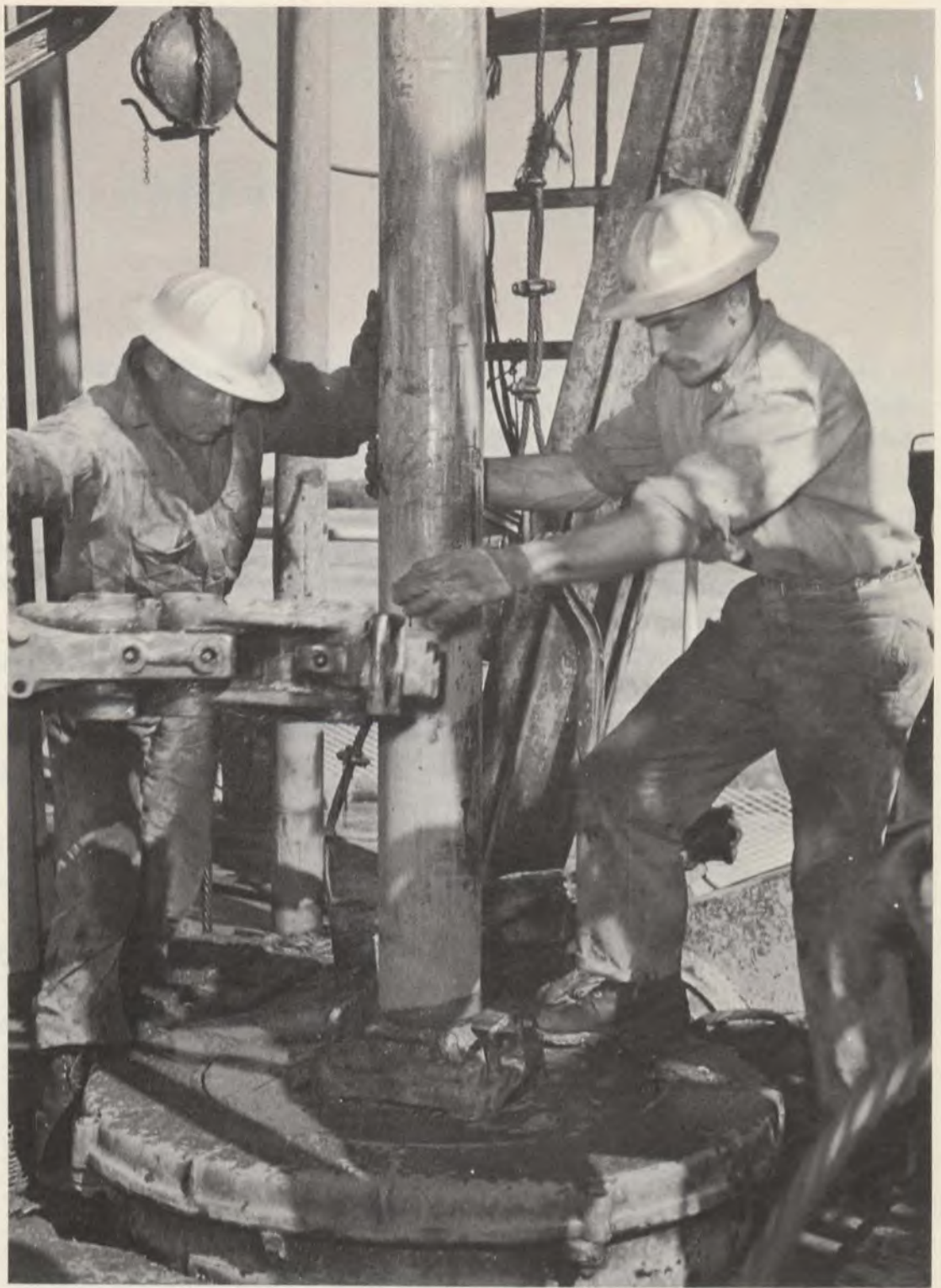
Workmen join pipe ends, called "spinning it in", at the Imperial Oil Ltd. fields north of Edmonton, Alberta.
