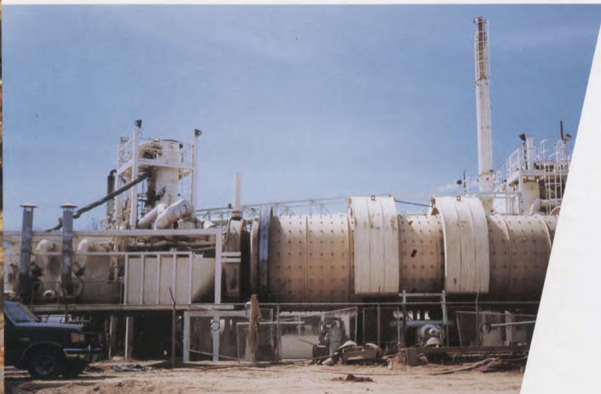
UMA Engineering Ltd. – Aostra Taciuk processor for clean-up of P.C.B. contaminated soils.
