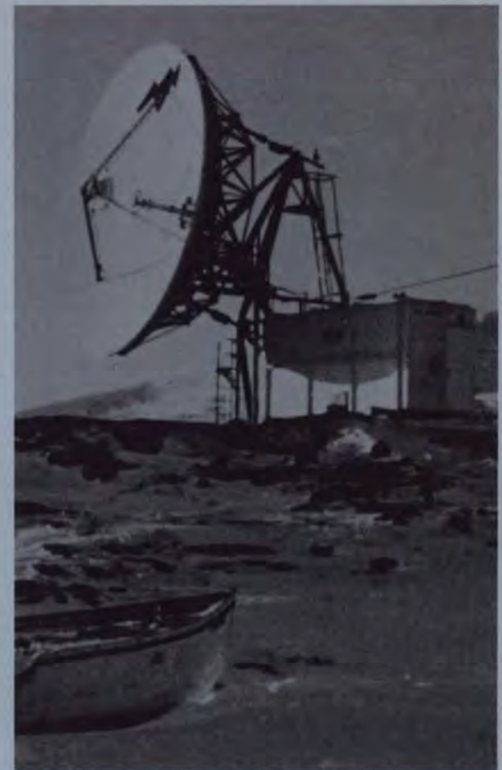
The Telesat earth station at Pangnirtung, N.W.T., Lat. 67 degrees N., provides telephone, radio and television services to the native communities in Baffin Island.
