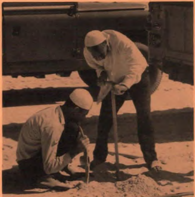
Soil testing for the international airport in the Trucial States, Sheikhdom of Abu Dhabi, an oil-rich state in the Arabian (Persian) Gulf.
