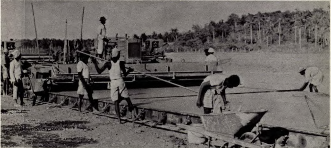
Laying concrete by machine for the main runway of the Katunayake airport development programme in Ceylon. The rails on which the machine rides also make up the forms to contain the new concrete.
