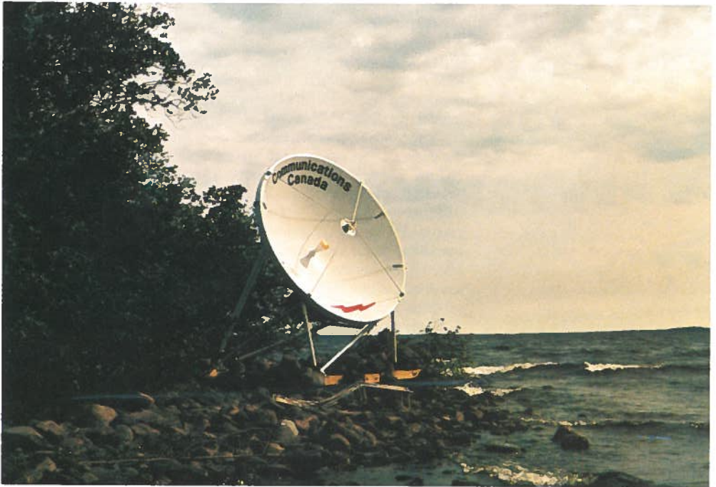
Telephony earth station, on shores of Black Lake, Sask., links remote mineral exploration site via satellite with Calgary head office. Photo: Canadian Petroleum Association
