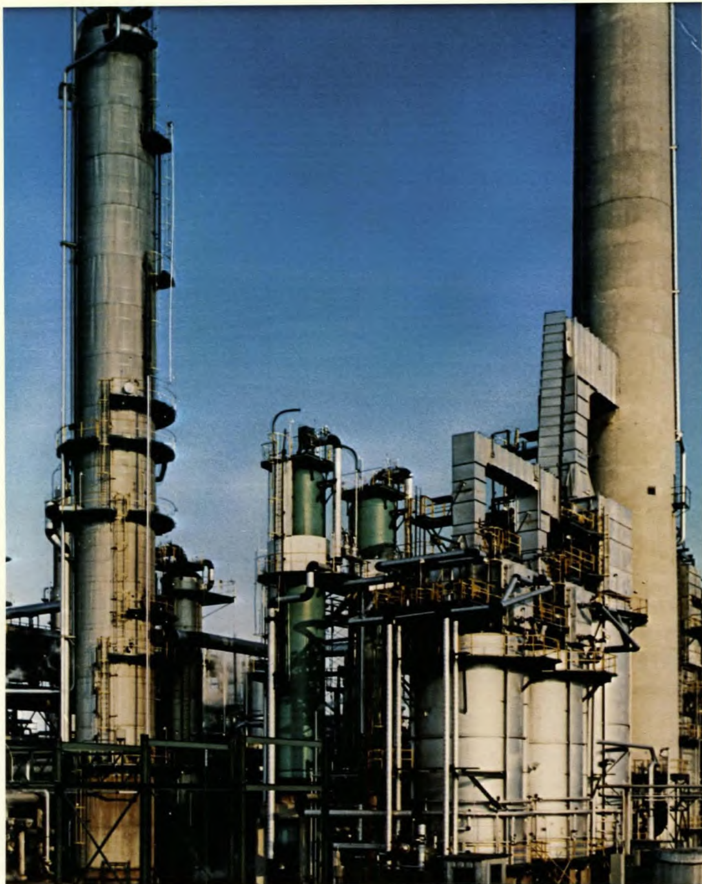
Mixed feed hydrofiner which, along with other major units such as a hydrocracker, powerformer, cryogenic hydrogen purification unit, hydrogen synthesis unit and light ends revamp, comprises a $50 million refinery expansion for Imperial Oil Limited at Sarnia, Ontario.
