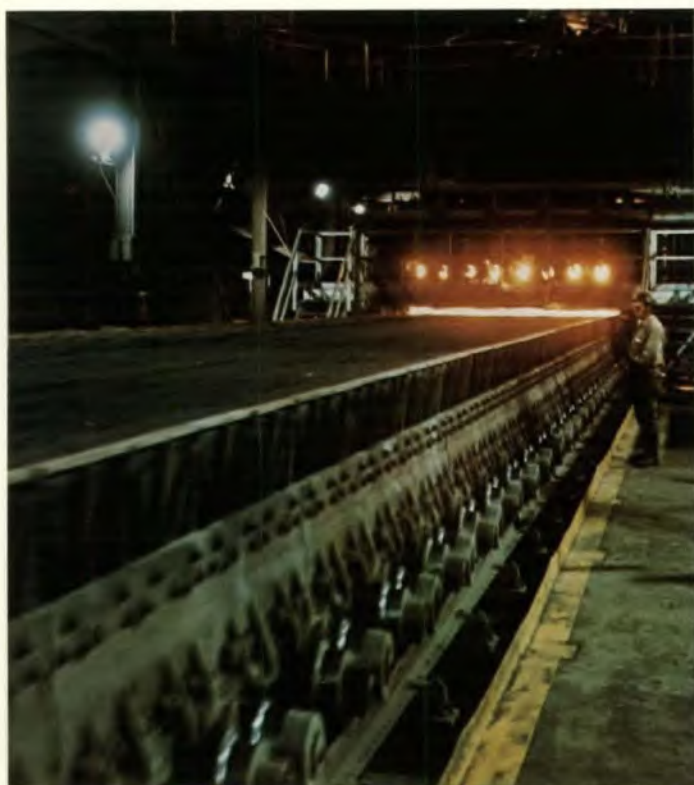
Complete sintering plant, including facilities for raw materials storage and handling, preparation and dust collection. Engineered and constructed for the Algoma Ore Division of The Algoma Steel Corporation at Wawa, Ontario.
