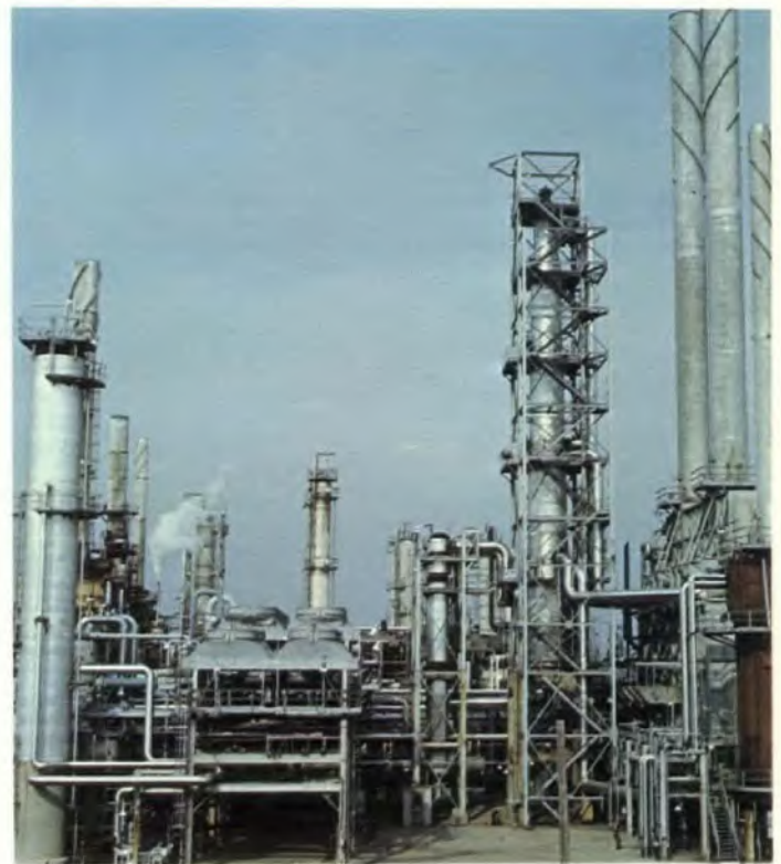
20,000 BPD catalytic reformer process unit constructed at the Montreal East refinery of Shell Canada Limited.
