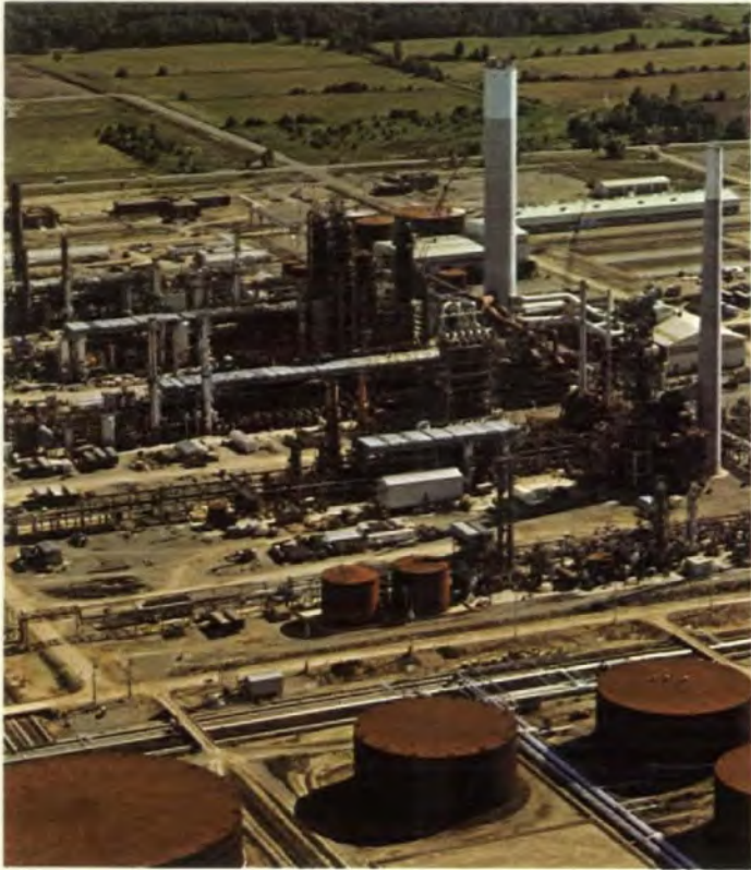
Construction for a 100,000 barrels per day refinery being built for Texaco Canada Limited at Nanticoke, Ontario.
