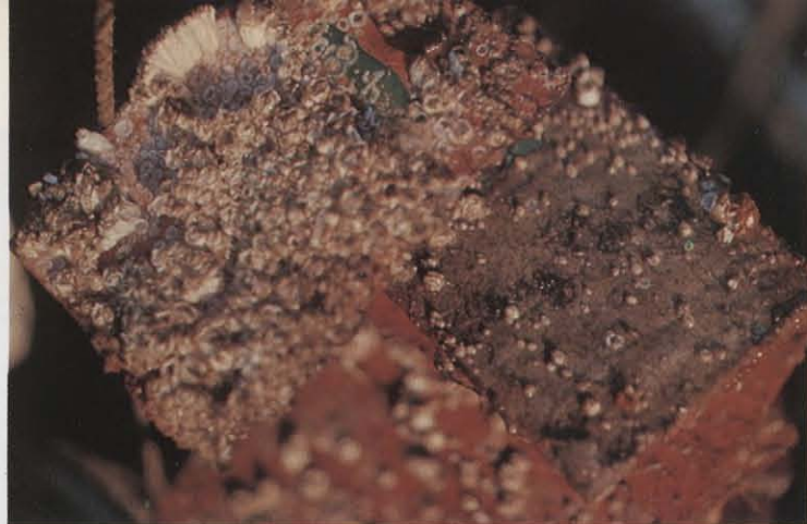
BARNACLE CONTROL — Barnacles grow luxuriantly in B.C. waters causing fouling of boats and marine structures. An anti-barnacle coating (right quadrant) shows promising effects.
