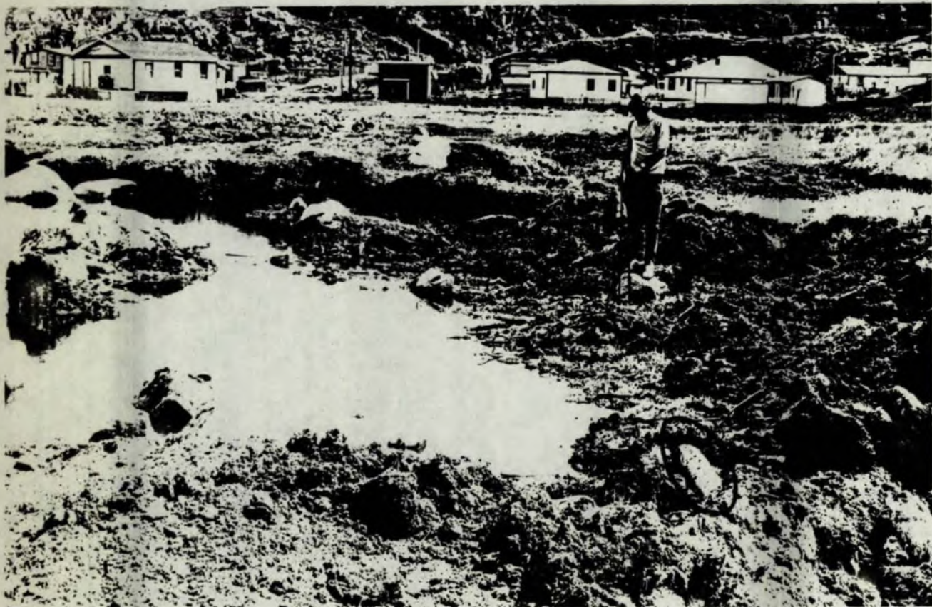
PHOTO NO. 2 Exposed pipe in school yard area. A man standing on a rock which rests directly on the pipe.
