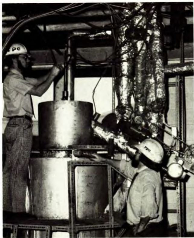
Adjusting Compressed Air Operated Liquor Spray Gun in Reactor
