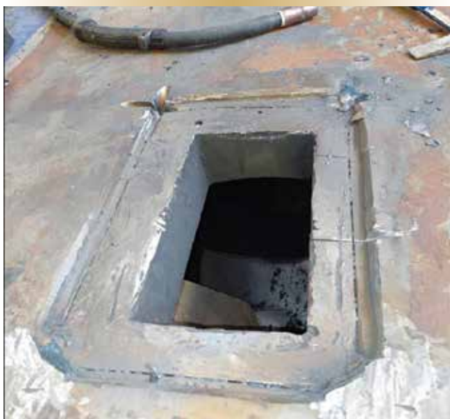
Figure 2. Port-side keyway window with cover plate removed to access the wedges. Gouges from the rotary saw are visible in the rudder hub casting.
