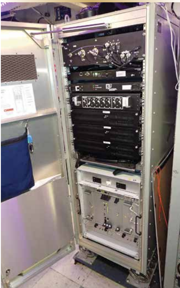
The ICTRS base station.
