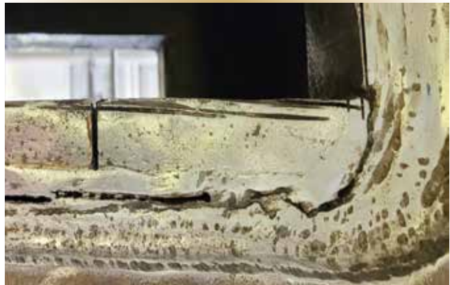
Figure 6. Starboard-side keyway window – pre-existing defects caused by a rotary saw and plasma torch, discovered May 19, 2022.
