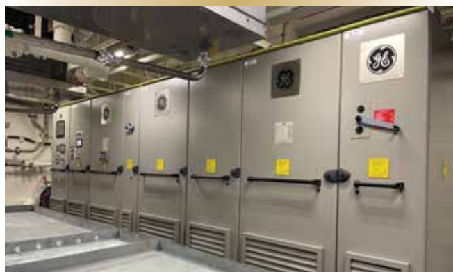
Figure 1. Converter cabinet in the starboard upper motor room aboard HMCS Margaret Brooke (AOPV-431).
