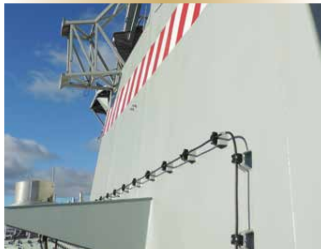
The DAS Rx Extension cable run topside.
