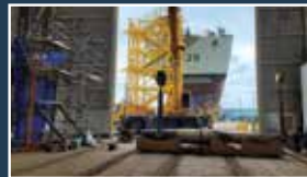
HMCS Charlottetown on the Halifax Dockyard Syncrolift for rudder repairs. (Photo courtesy FMF Cape Scott)
