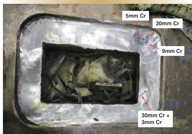
Figure 4a. Port keyway– MT defects discovered (May 6, 2022) following weld material build-up repair.
