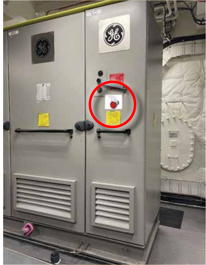
Figure 3. The cabinet with a mocked-up exterior logic reset pushbutton affixed.
