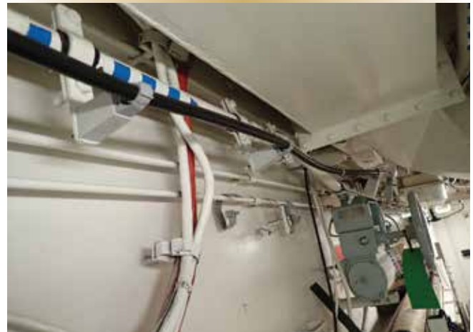
The (black) cable run for the distributed antenna system through the Gunners Stores flats.
