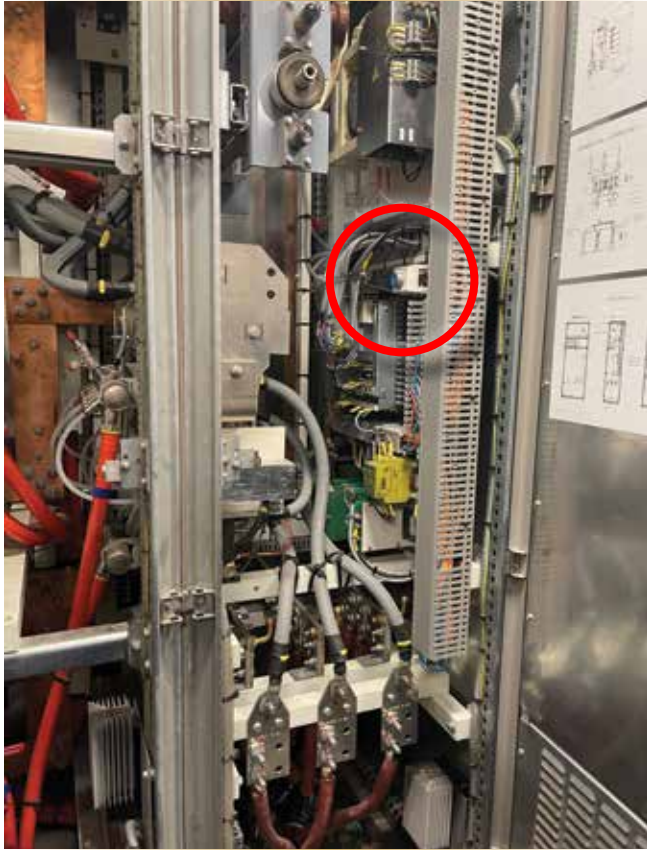
Figure 2. Current location of the logic reset button inside the ILC converter cabinet.
