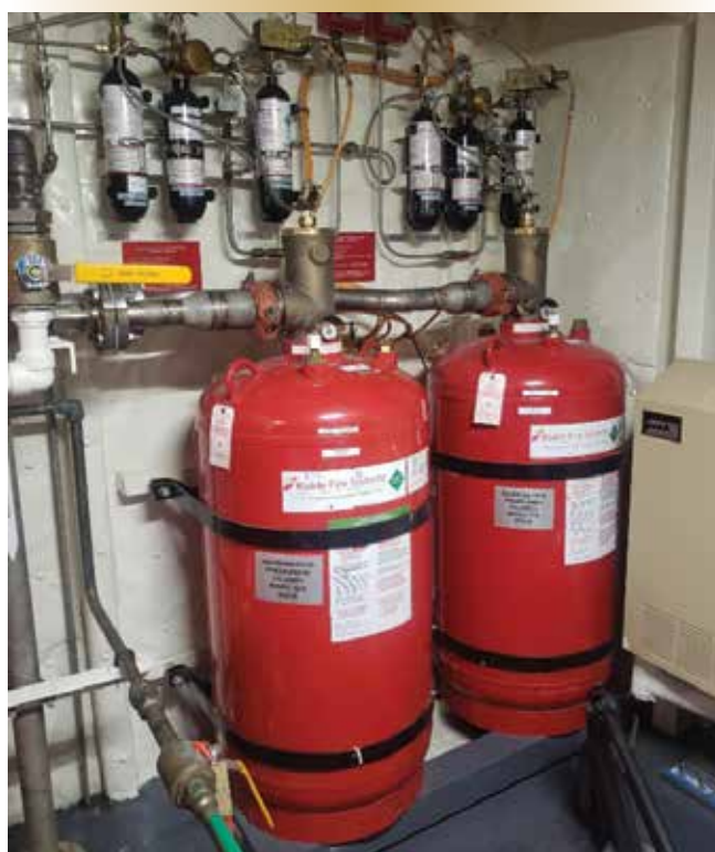
Figure 1. Novec 1230 arrangement on board HMCS Harry DeWolf for the port/starboard LV (low-voltage) spaces.
