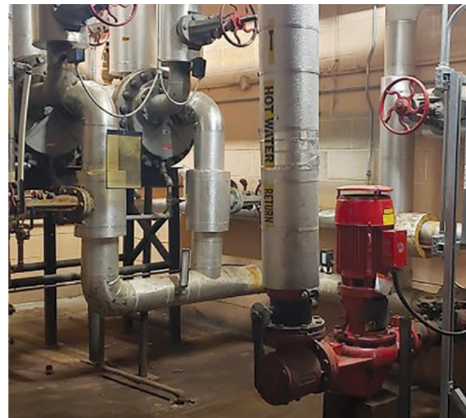
This hydronic heat distribution system was retrofitted at CFB Kingston to decrease energy consumption and fossil fuel dependence, as part of the IDEaS Green Heat challenge.
