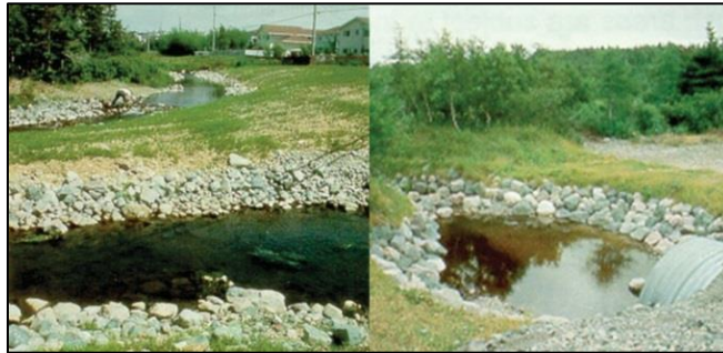
Figure 37. Photos of stream bank vegetation (hydroseed) and rip rap (left). Rebuilt stream banks using rip rap, sod and natural vegetation (right)
