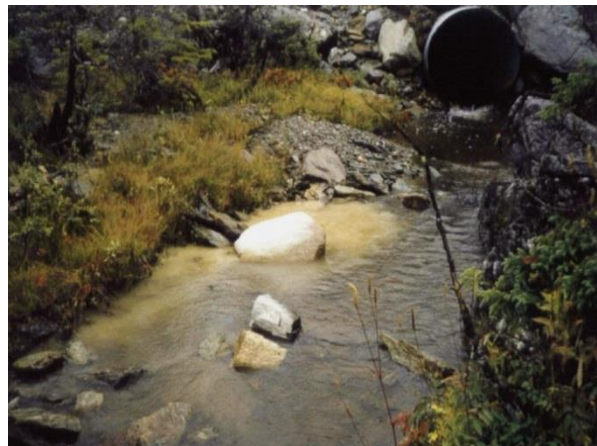
Figure 12. Visible sediment entering a stream near a road crossing
