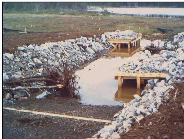
Figure 33. Constructed instream cover (undercut lunker structures (right) and rootwad placement (left)) in a man-made stream prior to re-watering
