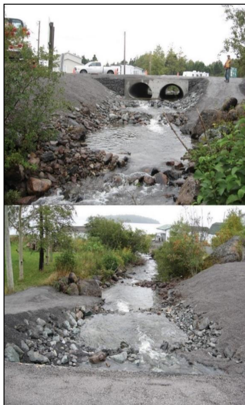
Figure 45. Culvert with tailwater pools
