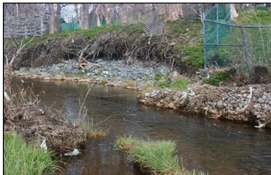
Figure 41. Collapsed gabion structure has decreased stream width and has caused excess erosion directly downstream
