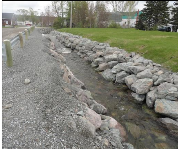
Figure 9. A highly impacted channel and banks next to a road
