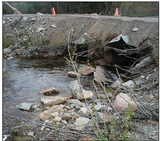
Figure 47. Proper pool construction but poor bank protection
