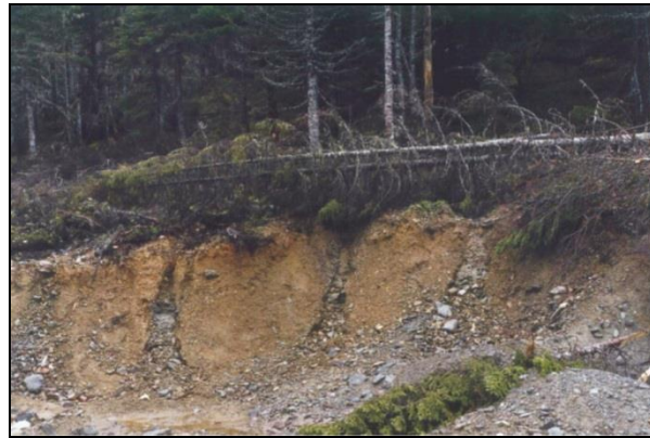
Figure 21. Excessive streamside erosion
