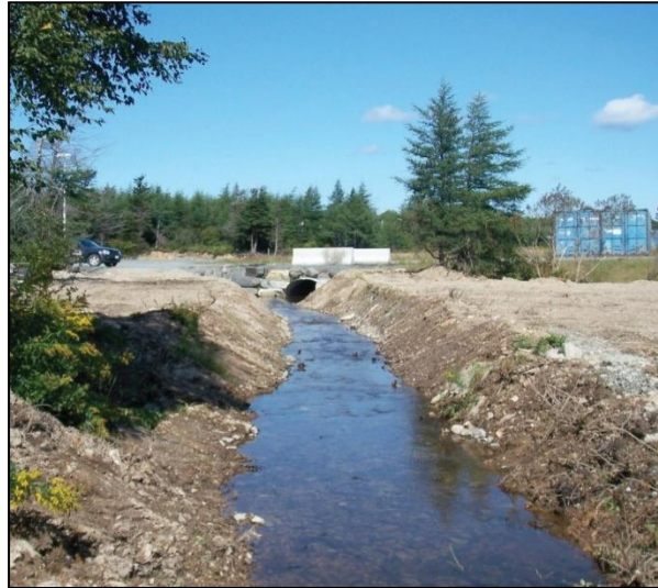
Figure 10. Channelized stream showing loss of vegetation
