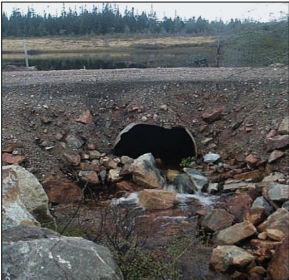
Figure 46. An ill attempt to create a plunge pool on an improperly installed culvert
