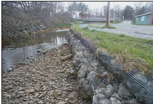
Figure 40. Typical stream bank gabion (note backfill and planted grass to assist in stabilization)
