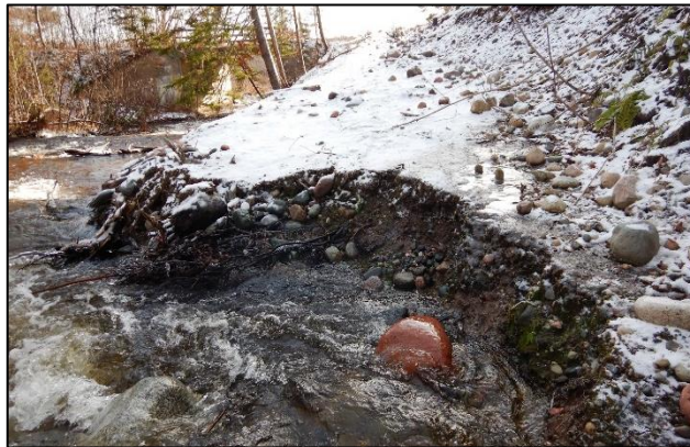
Figure 14. Stream bank showing a large amount of erosion and altered water flow
