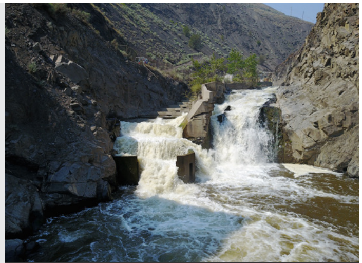
The damaged Bonaparte River fishway in 2018. Photo credit: DFO Staff.
