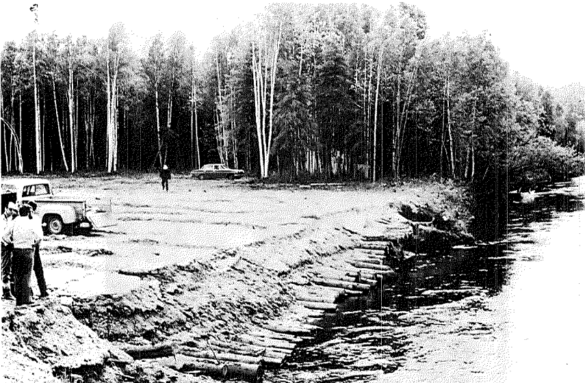
Fig. 10. Chatinika River crossing, near Fairbanks. Note logs used as riprap and erosion of river bank after only four months.
