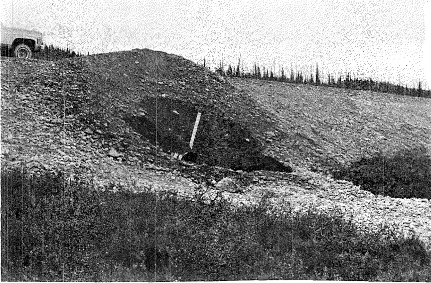
Fig. 22. Inadequate side slope drainage will result in failure of haul road.
