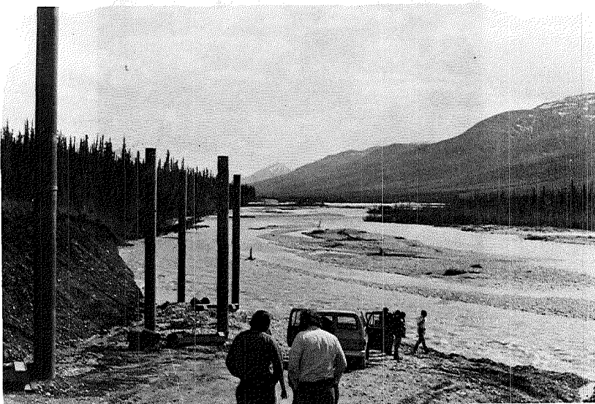
Fig. 17. Vertical-support-members in place to bank of Dietrich River. Pipeline was scheduled to be built through prime grayling overwintering area until JFWAT intervention.
