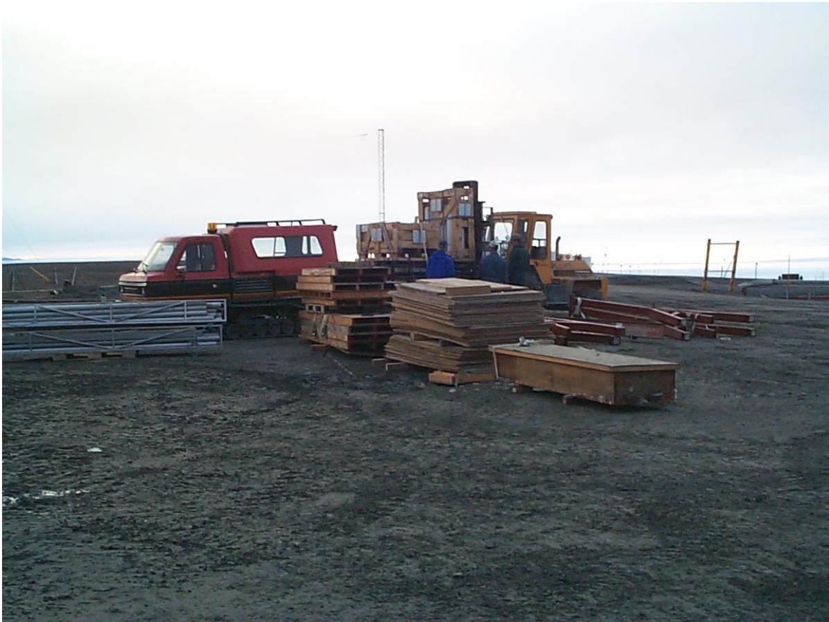
Figure 140: Clean-up work at CFS Alert in the cool, wet, and muddy conditions typical of summer's melt in the Arctic. Photo credit: Al Tremblay.
