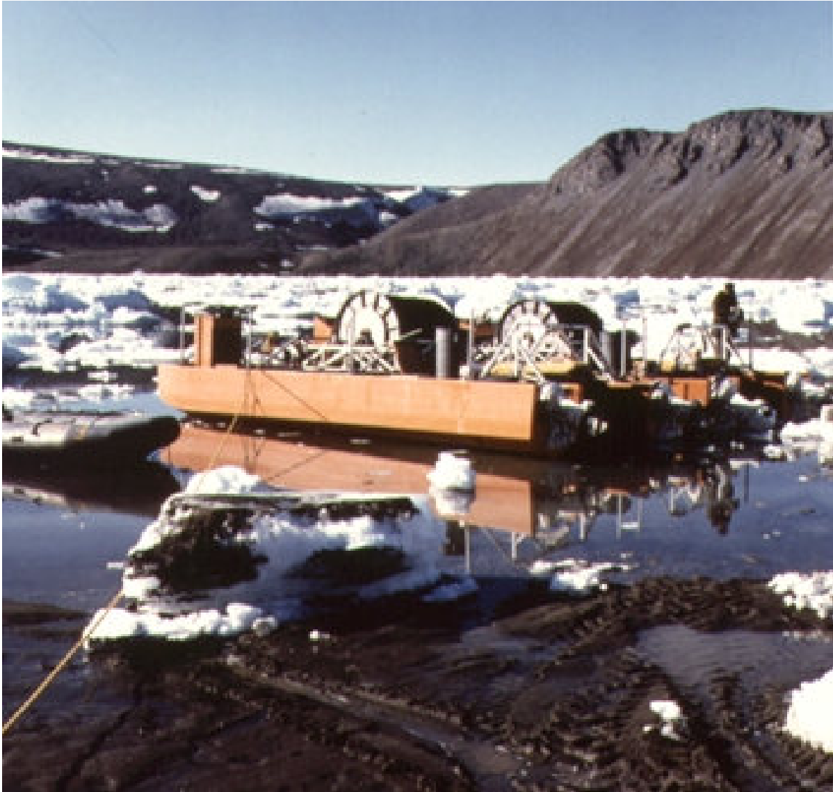
Figure 86: The two cable-laying catamarans in an ice-choked Wrangel Bay. The operators had to wait until the ice had been blown out of the Bay before they could lay the hydrophones and the cable. Photo credit: DRDC.
