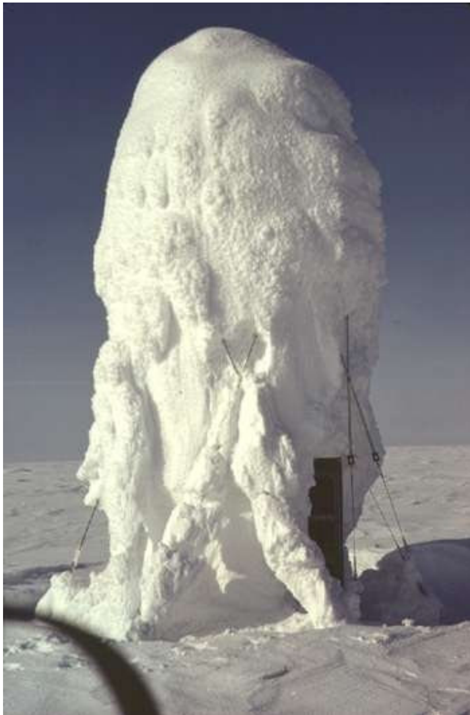
Figure 91: Silo showing the frost that had collected on it during the preceding winter. Photo credit: DRDC.
