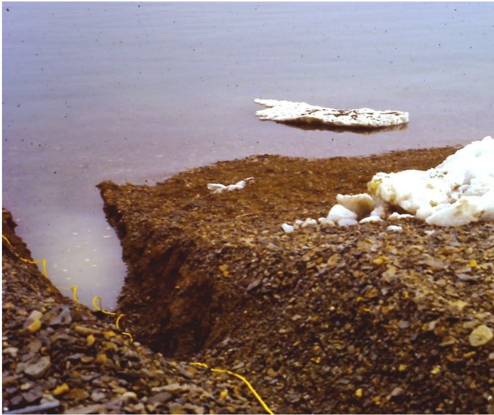
Figure 113: A trench through the foreshore. Note the yellow cable. It was buried later. Photo credit: Ron Kuwahara.
