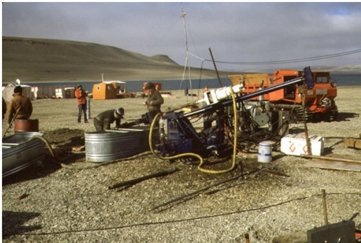
Figure 93: Drill rig drilling slanted hole at Gascoyne Inlet. The hole passed through the gravel and rock and entered the water through the sloping bottom. Photo credit: DRDC.
