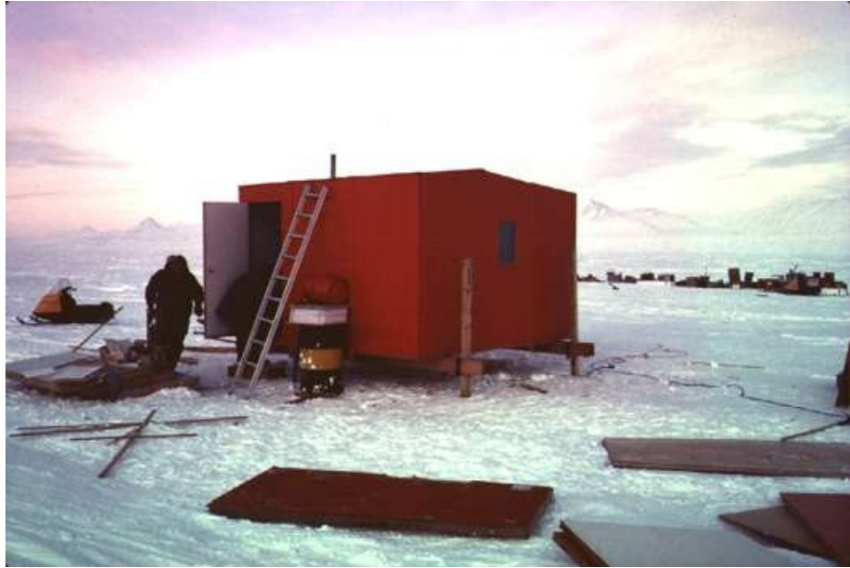
Figure 105: A building under construction on the Ward Hunt Ice Shelf. Note that the pilings supporting the building are sitting on top of the ice. They were melted down into the ice later. Photo credit: DRDC.
