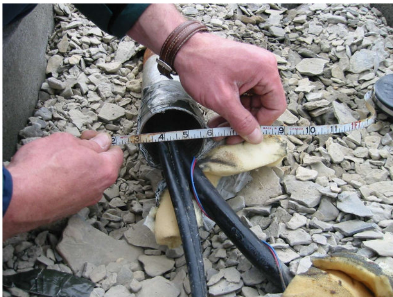
Figure 94: The shore end of the pipe that is casing the hole. This picture was taken in 2009. Photo credit: DRDC.
