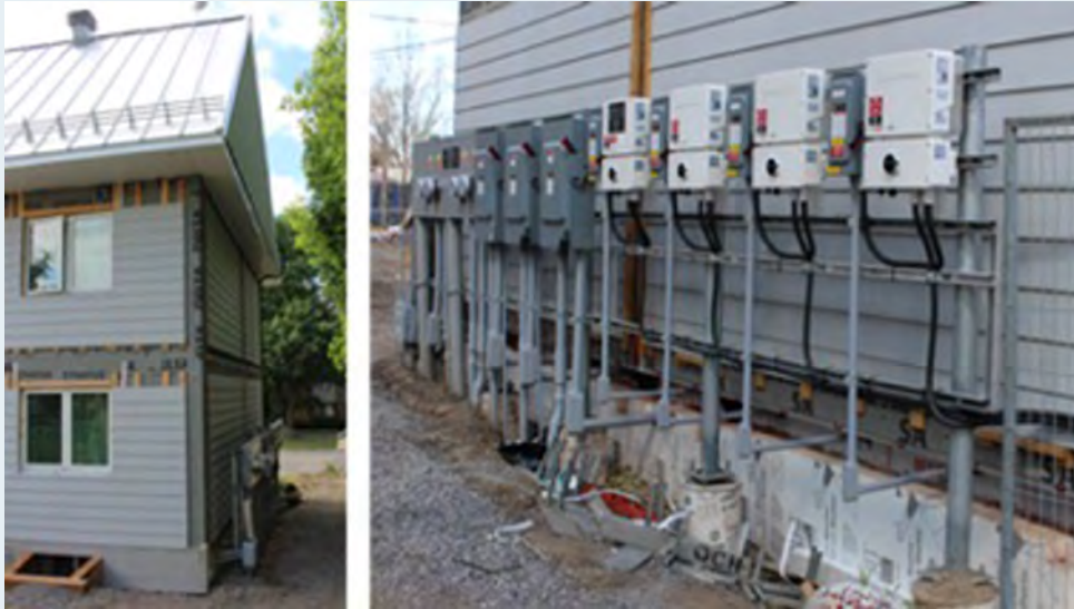
Figure 3-10: Ottawa Community Housing electric infrastructure mounted on racks anchored to piers stood-off sufficiently from building to allow panels to be installed behind.
