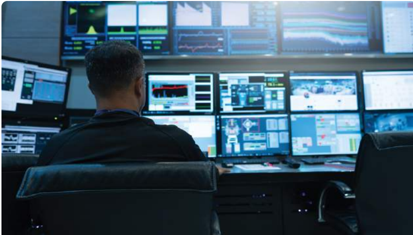
Aligning operation schedules with actual building use Optimizing the sequence of operation for building systems
