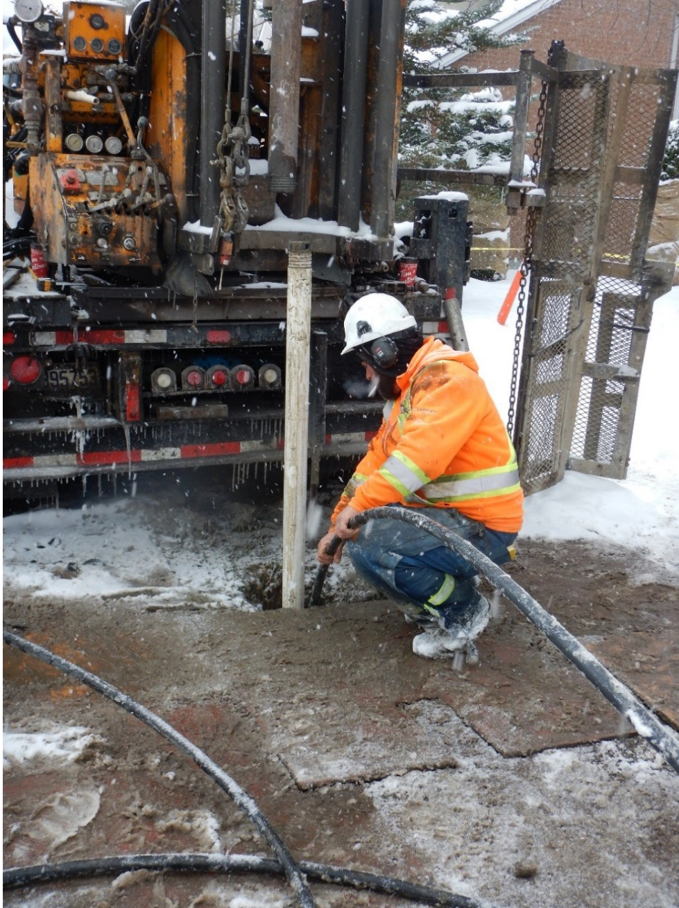
Figure 15. Filling the borehole annulus of GSC-VC2 with grout pumped through a tremie pipe after removal of the drill casing; Photograph by M.J. Hinton; NRCan photo 2022-337
