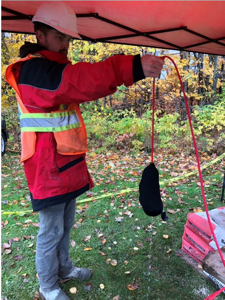
Figure 16. Vibrating wire piezometer packed in filter sand prior to installation at BC16; Photograph by M.J. Hinton, NRCan photo 2022-338
