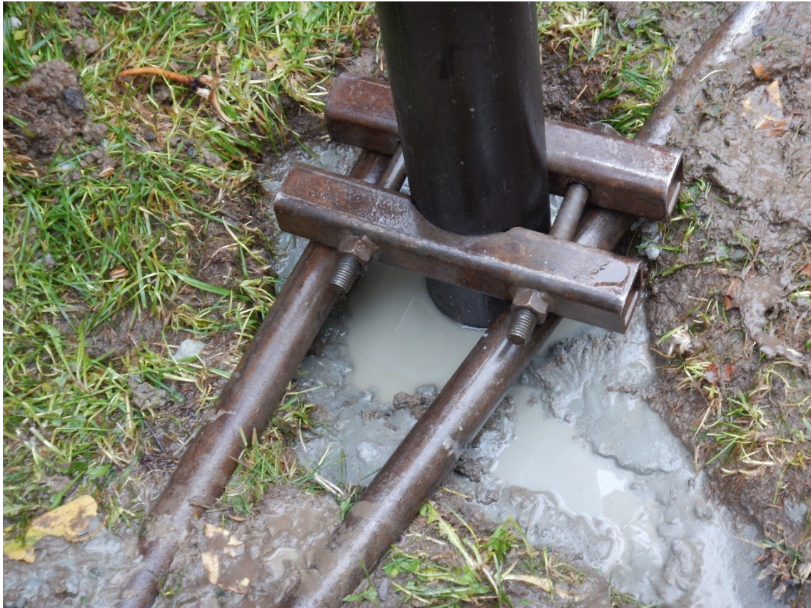
Figure 13. Clamp attached to drill casing and supported by two, A-sized, drill rods; Photograph by M.J. Hinton, NRCan photo 2022-335
