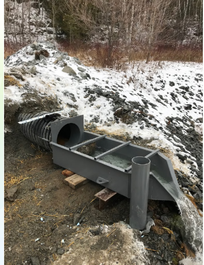
H-Flume at Shaft #98
