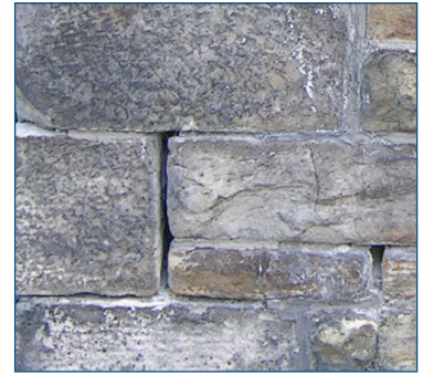
De-bonded Masonry Unit [2]
