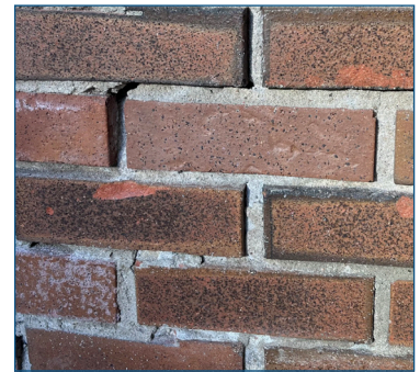
Fire Skin Damage
