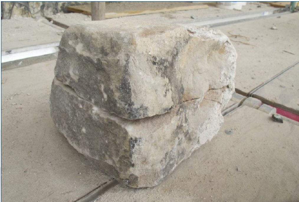
Figure 15: Cracked masonry unit due to freeze-thaw damage [2]
