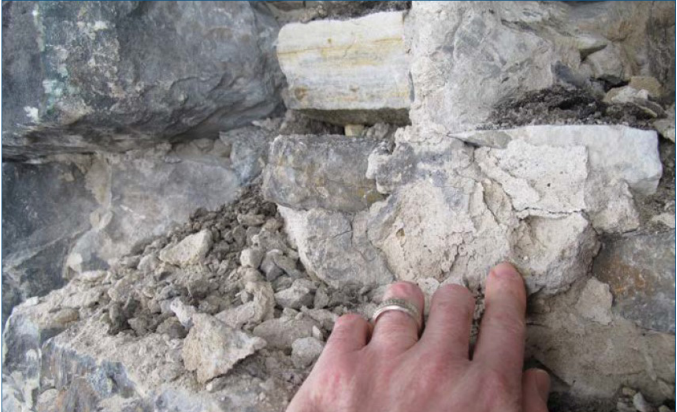
Figure 16: Cracked masonry unit due to freeze-thaw damage [2]
