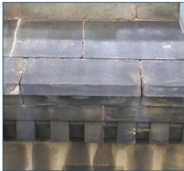
Open Masonry Joint [2]
