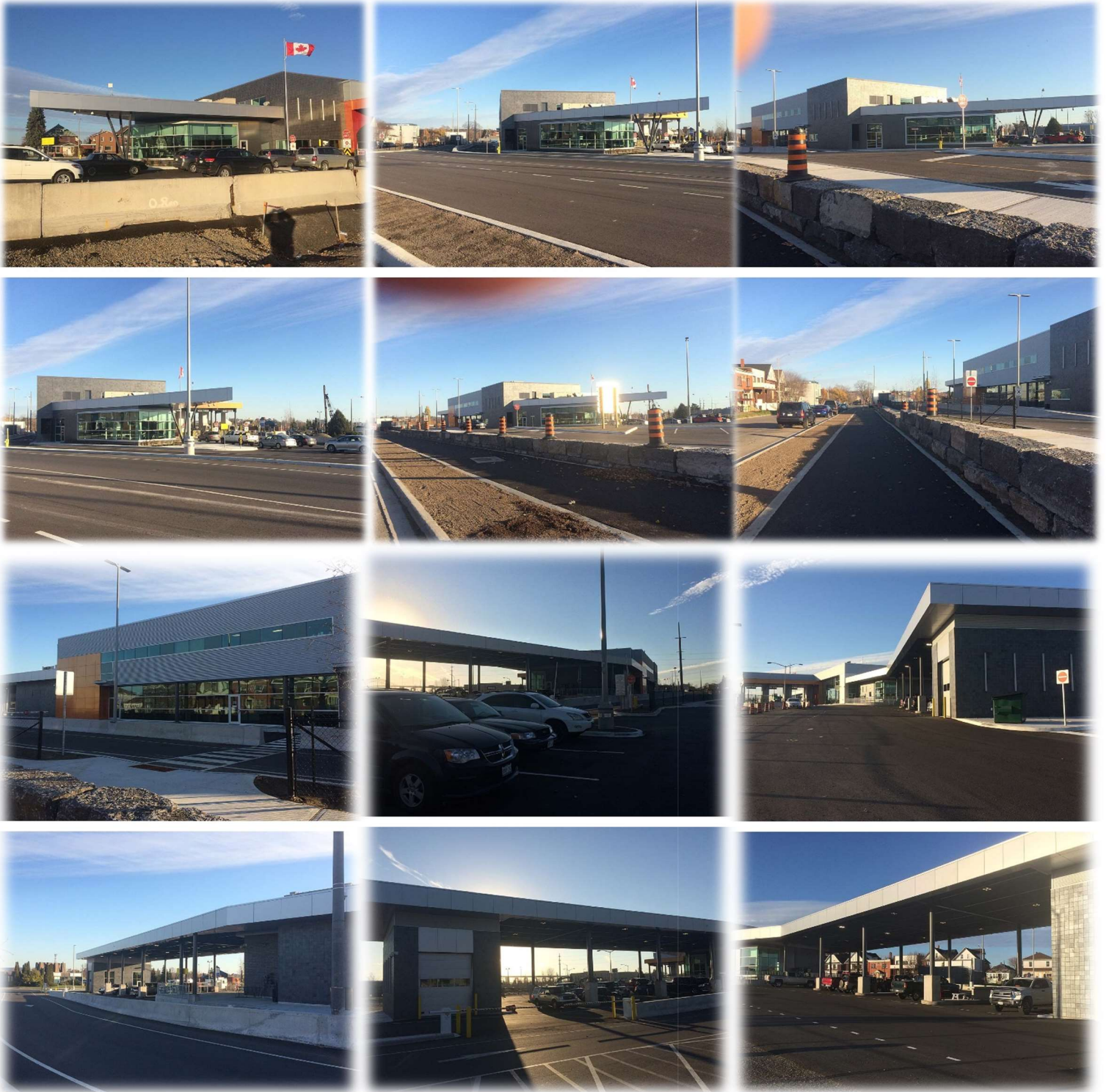
b) Work progress at the Canadian Plaza Redevelopment in Sault Ste. Marie
