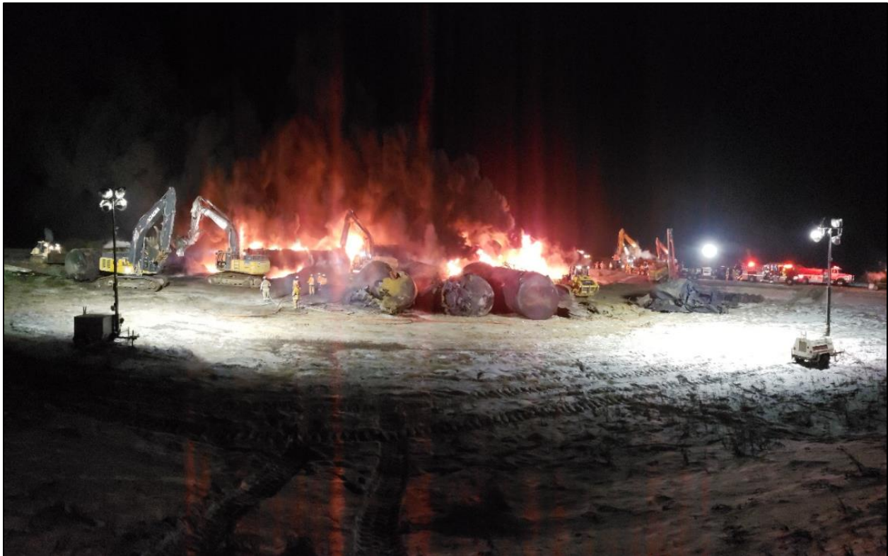
Figure 19: View of incident described in TSB R19W0320
