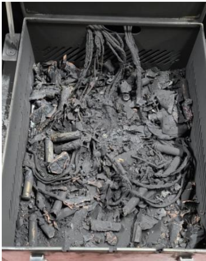
Figure 18: B2 Sample 13, 14, 15, 16 – T.7 photographs showing a lot of debris from the explosion
