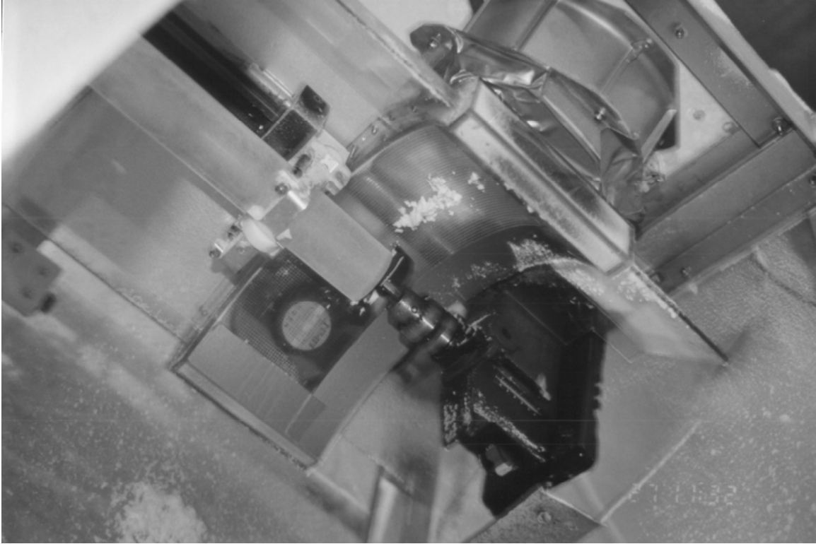
Photo 2.7 Snow Distribution Plenum
